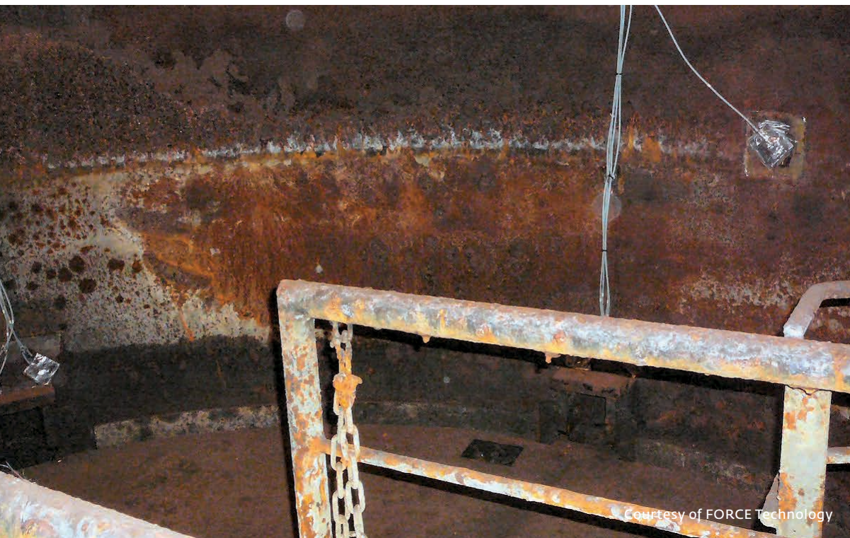
Corrosion inside a wind turbine
