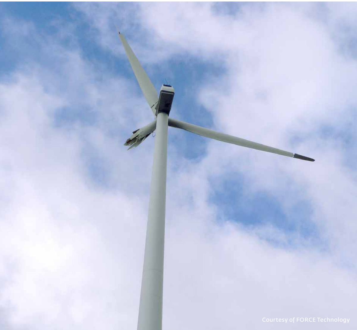
Blade collapse after failure of the load bearing structure
